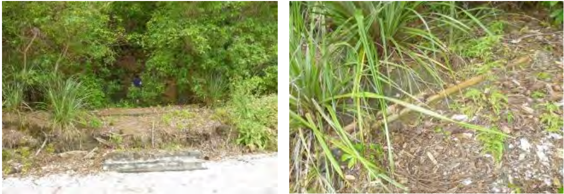
Figure 106 Boatshed cut into cliff and b) drain Source: Auckland Council Heritage Unit
