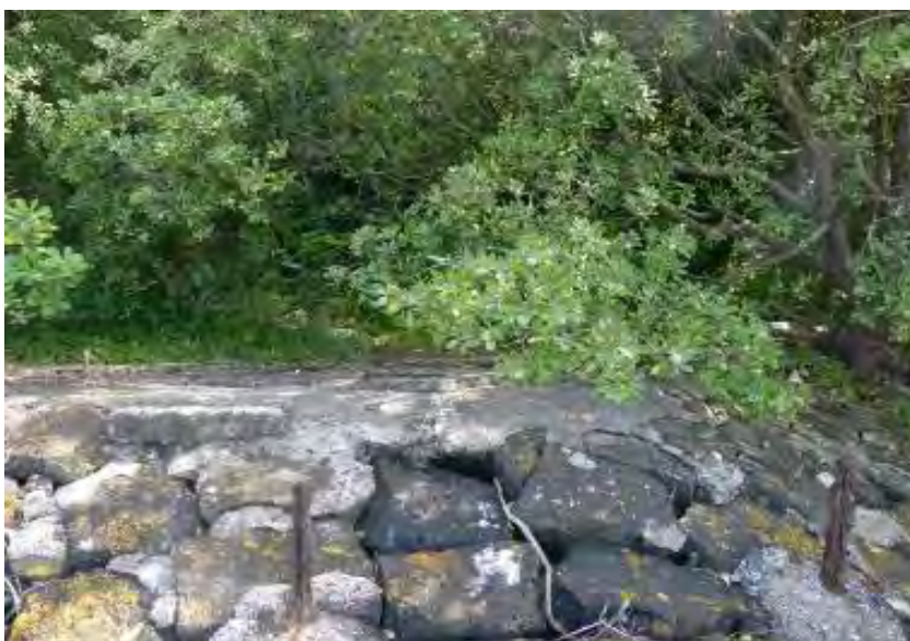
Figure 78 a & b Views of mid 1920s Septic Tank Auckland Council Heritage Unit January 2014
