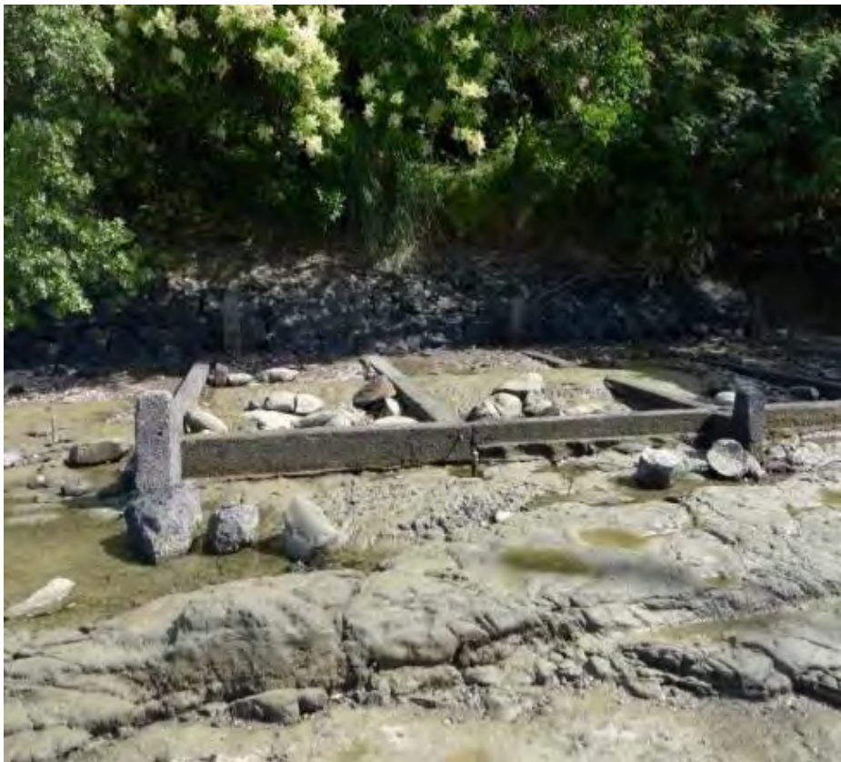
Figure 77 a & b Two views of foundations of 1959 Boat Shed Auckland Council Heritage Unit, January 2014
