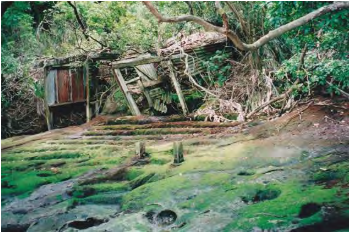
Figure 87 Wesley Bay Boatshed note two posts also shown in figure 85. Photograph taken by Cuni de Graaf prior to its final collapse.
