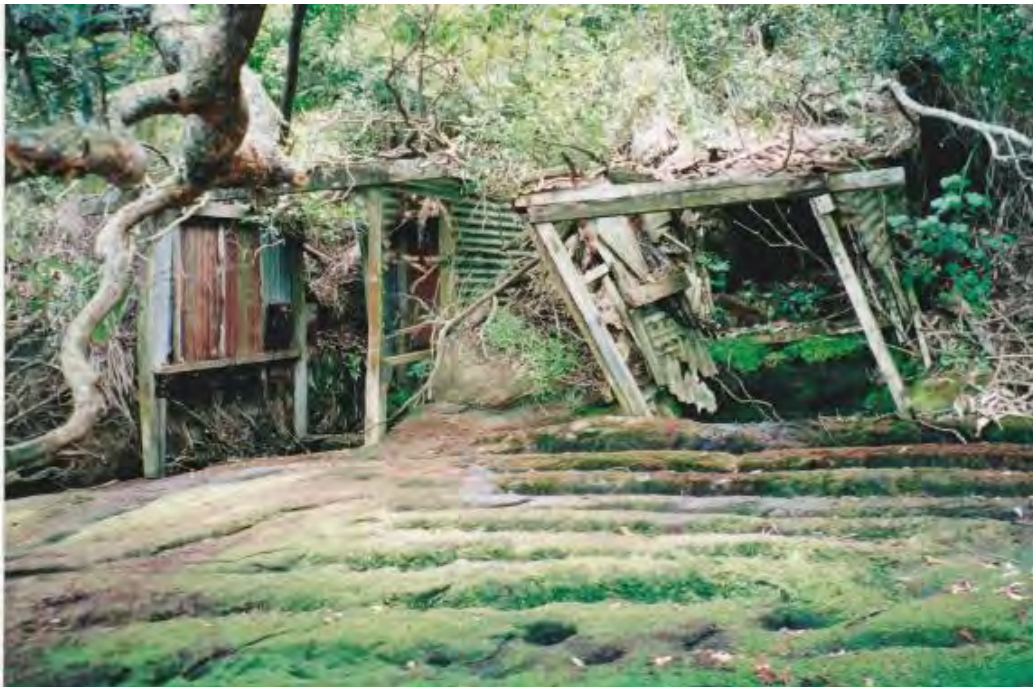
Figure 88 Another view of Wesley Bay Boatshed prior to collapse. Photograph Cuni de Graaf.
