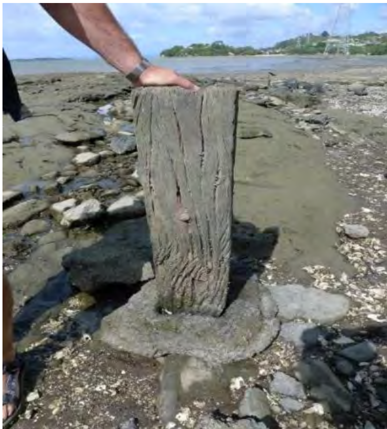
Figure 79 Remains of pipeline from Septic Tank to Manukau Harbour, Source: Auckland Council Heritage Unit
