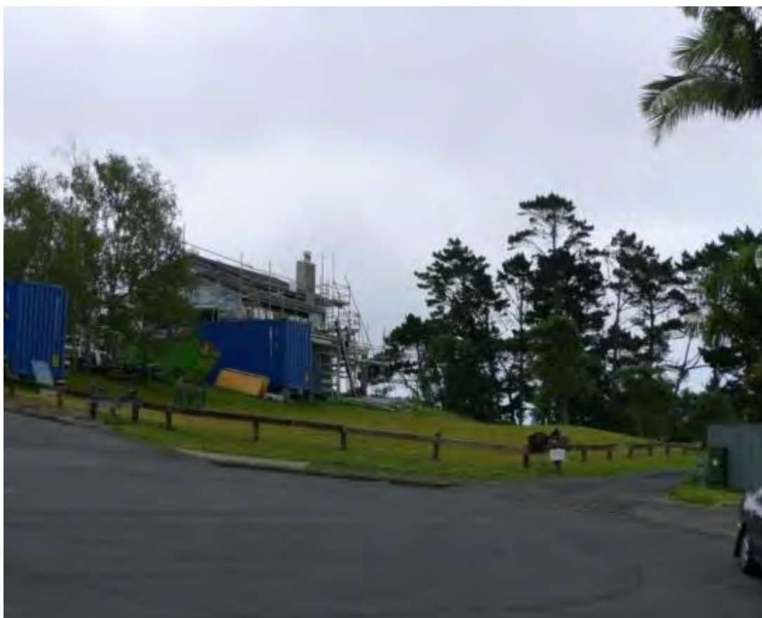
Figure 97 New construction in vicinity of former pa R11/100, Source: Auckland Council Heritage Unit
